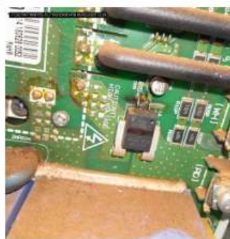
PCB inverter compressor 1
