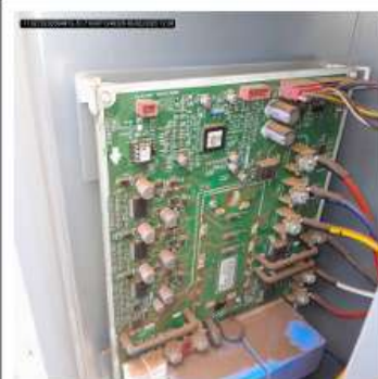
PCB inverter compressor 1
